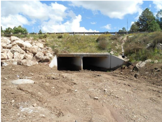
Caption-This is a part of the Sinclair Wash Trail where surveying and inventory took place. This is near San Francisco Street.
