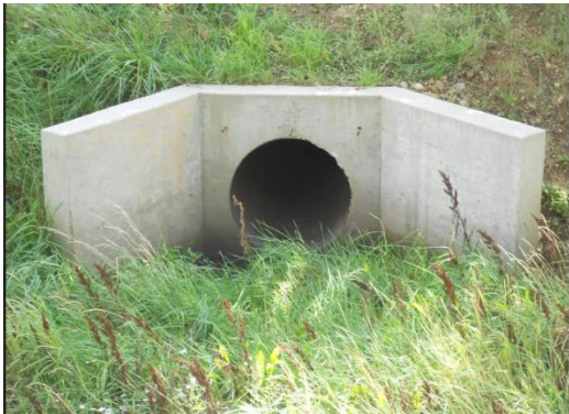
Caption- This is a culvert on the Sinclair Wash Trail. The pipe diameter was measured.
