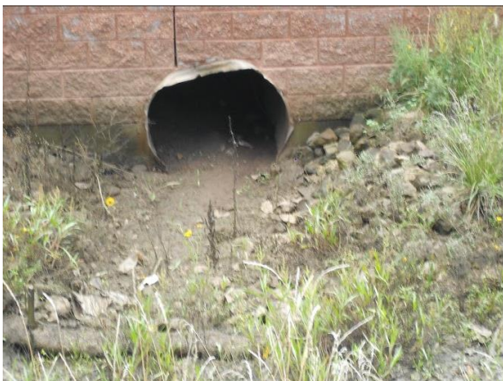
Caption- This is a part of the Sinclair Wash Trail where a pipe was measured.
