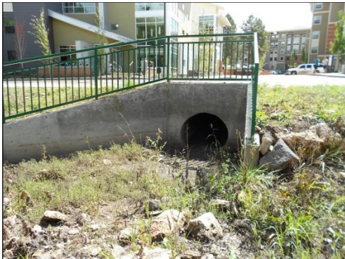
Caption-This is a part of the Sinclair Wash Trail where surveying was done near the Suites Apartments.
