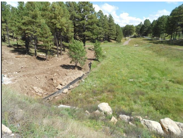
Caption-This is a part of the Sinclair Wash Trail where soil sampling and surveying took place. This is part of the Sinclair Wash Trail is heading towards the Grove Apartments.
