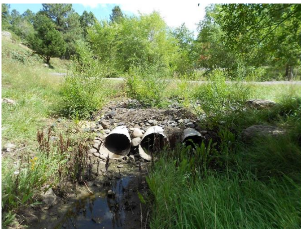
Caption-This is a part of the Sinclair Wash Trail where the pipe diameters were measured and plant inventory was taken.
