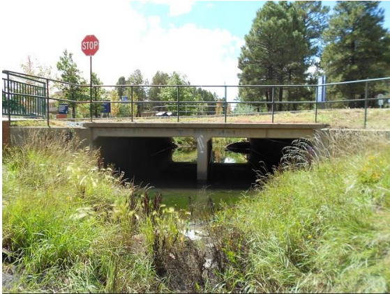
Caption-This is a part of the Sinclair Wash Trail on Northern Arizona University Campus. This is where the bridge goes from one cross section to another near the Suites Apartments towards Pine Knoll Drive.
