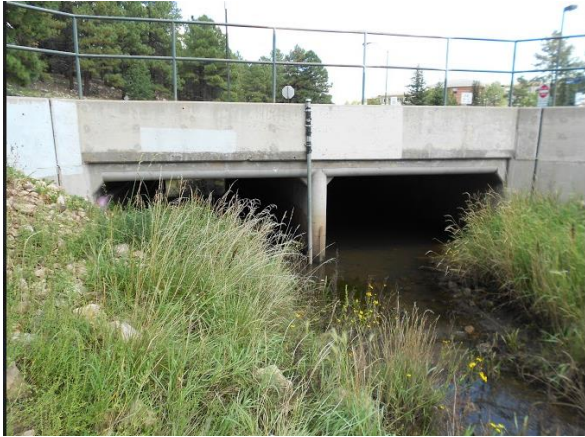
Caption- This is an underground tunnel that goes between cross sections on Northern Arizona University Campus for the Sinclair Wash Trail.
