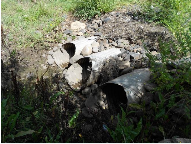
Caption-This is a part of the Sinclair Wash Trail where the pipe material inventory was taken.
