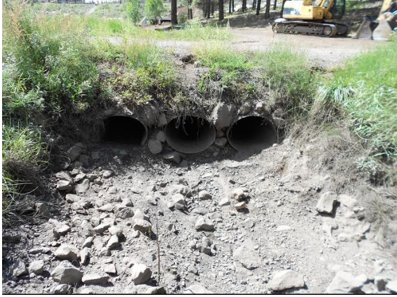
Caption-This is a part of the Sinclair Wash Trail where the pipe diameters were measured and inventory was taken.
