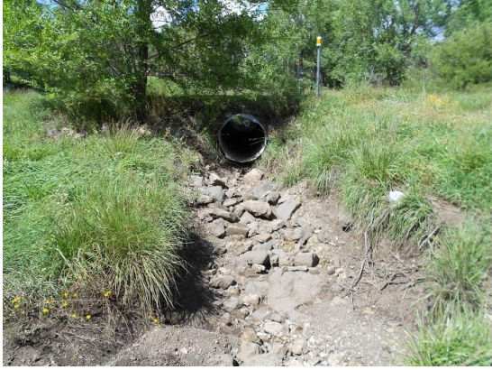
Caption- This a part of the Sinclair Wash Trail where plant inventory was taken and the pipe diameter was measured.
